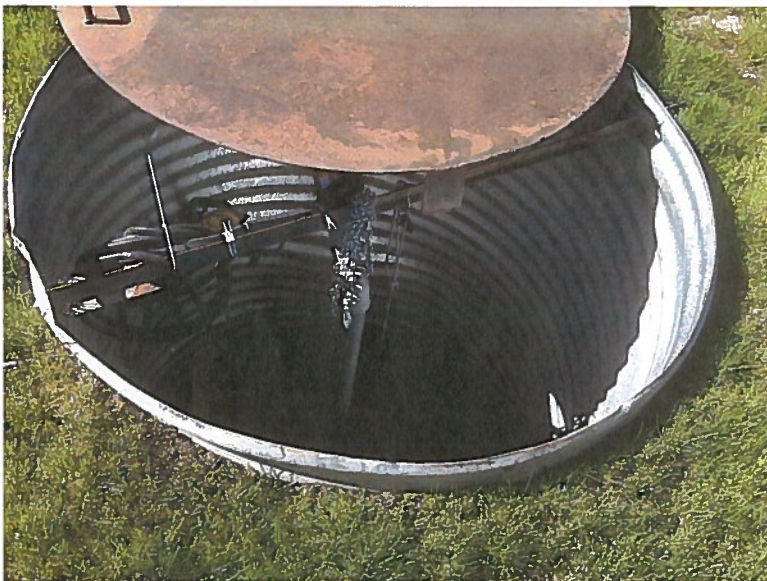
Pump Wet Well
