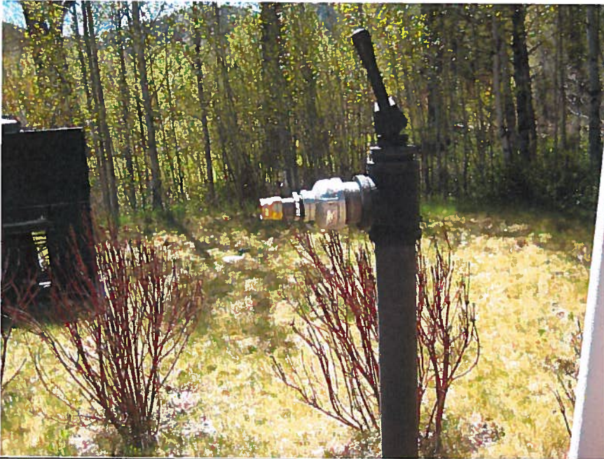
Hydrant with hose bib
