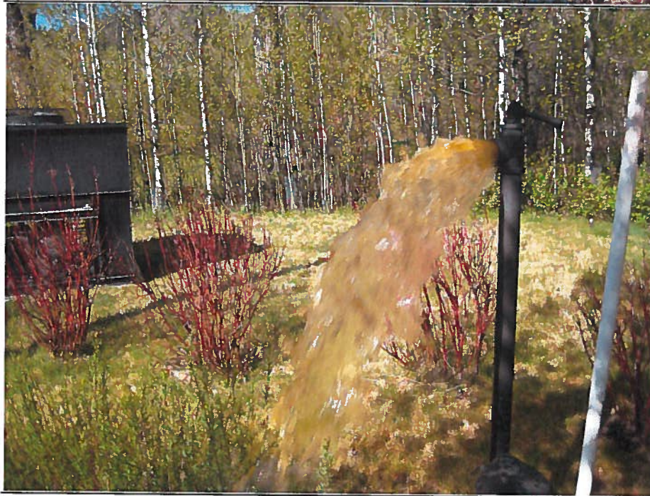
Hydrant before hose bib is attached
