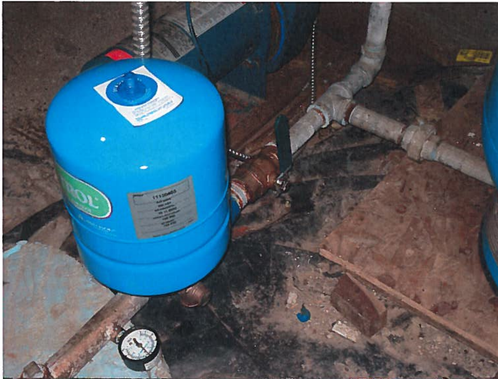
Pressure tank for the irrigation system
