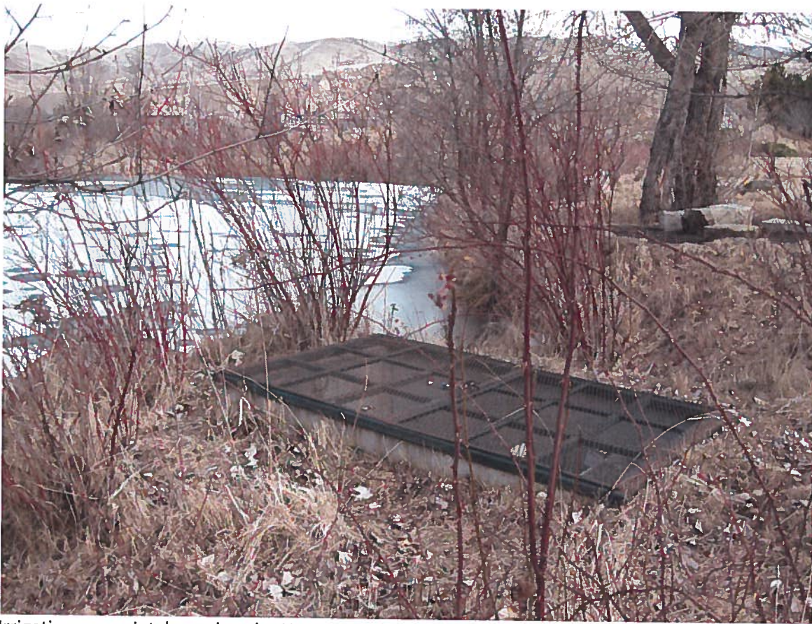
Irrigation pump intake and vault. Houses irrigation pump and flow meter.
