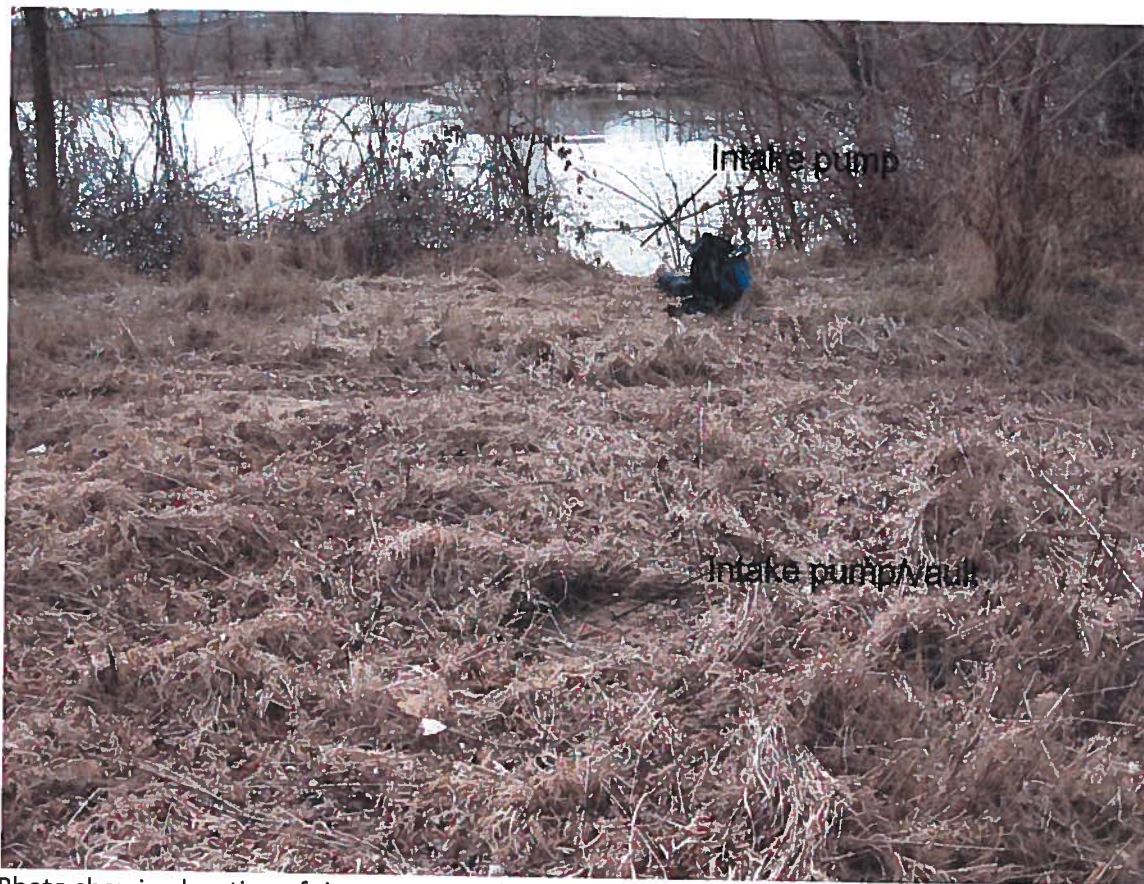
Photo showing location of river pump intake; pump in vault with vault in foreground.
