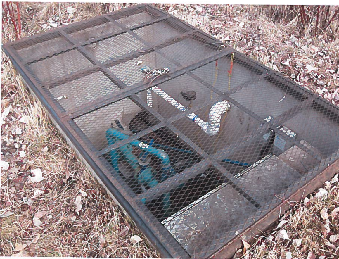
Irrigation pump and flow meter.
