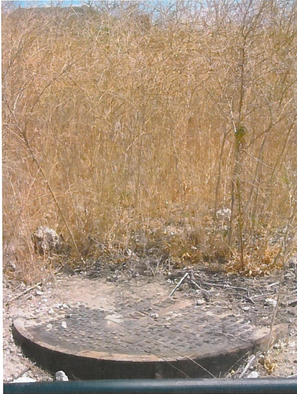
63-31877 License Exam 8/9/2011: Manhole cover with main line. Hook-up for each lot marked by a 2 x 4 board behind this manhole cover (difficult to see in this photo but at center in background). Pipeline and stubs buried 3 ft below the surface.
