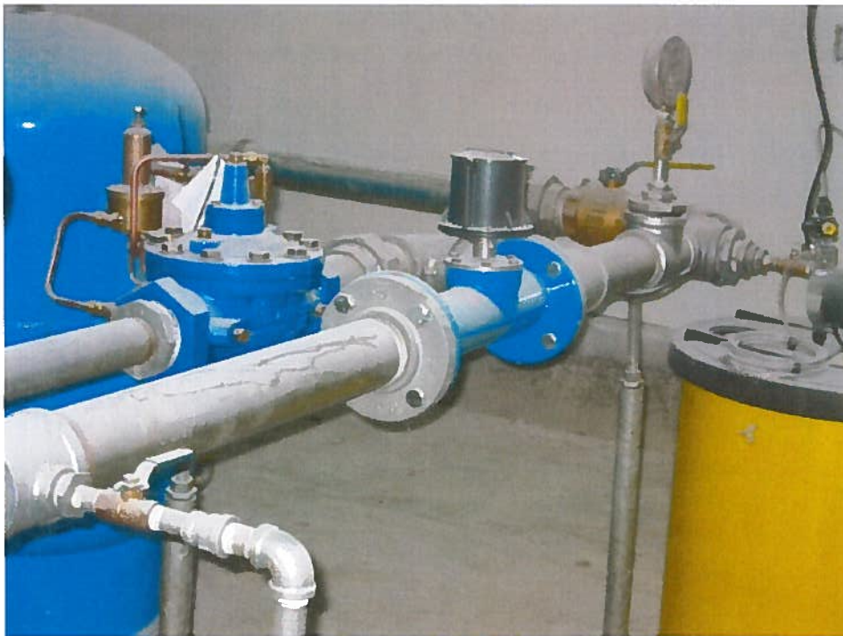
63-31877 License Exam 8/9/2011: Pipeline in well house from underground line from well to McCrometer flowmeter. Pressure gage then Chlorination tank (yellow) in place on line just after flowmeter. First of 3 pressure (bladder) tanks past elbow after chlorination tank.
