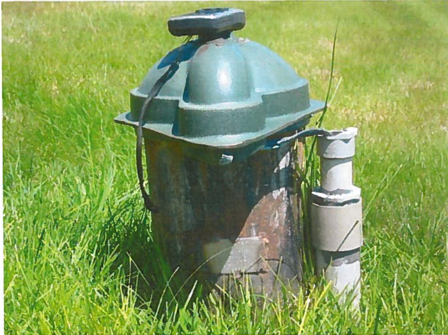
63-31877 License Exam 8/9/2011: Well (POD) with welded Tag #D0053122 facing north. Note well cap is not in place correctly. Well cap should cover top of PVC conduit with pump wires. This well drilled as a replacement well for Tag #D0042588.
