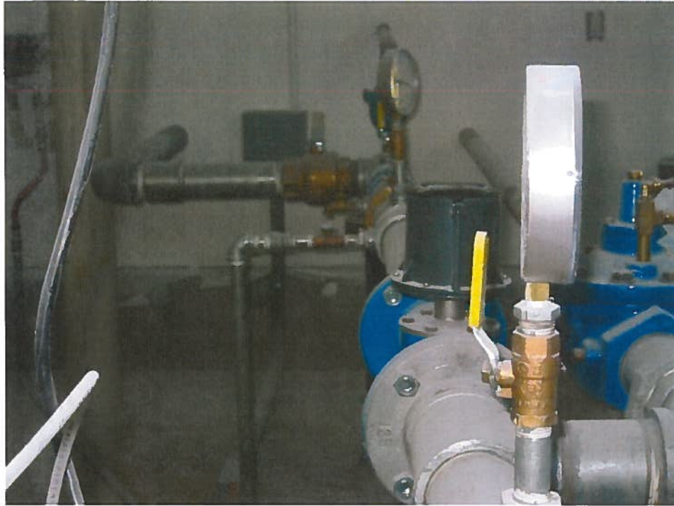
63-31877 License Exam 8/9/2011: Inlet pipe from well into pump house line. Pressure gage in place just before McCrometer flowmeter and second pressure gage before Chlorination system.
