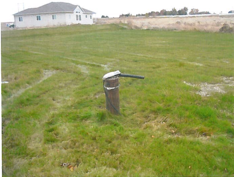
63-31877 License Exam 11/3/2011: Well with Tag #D0042588 facing east. Appears well likely to have pump in place per wires present and well lid that submersible pump capable of hanging from. Aluminum well cap sitting ajar on top does not meet well construction standards.
