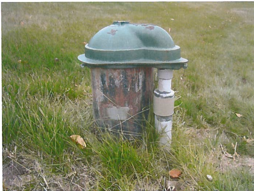
63-31877 License Exam 11/3/2011: Well (POD) with Tag #D0053122 facing north. Second site visit on 11/3/11 to verify condition of well with Tag #D0042588. Re-oriented well cap on D0053122 to correct position covering PVC conduit with pump wires per well construction standards.
