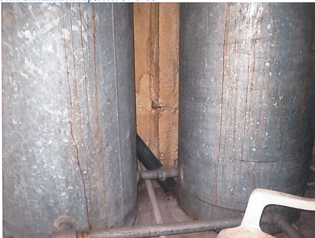
STORAGE TANKS ARE TIED TOGETHER
