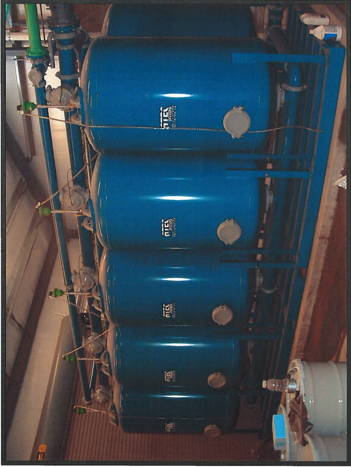
Water Treatment System – Pressure Filters
