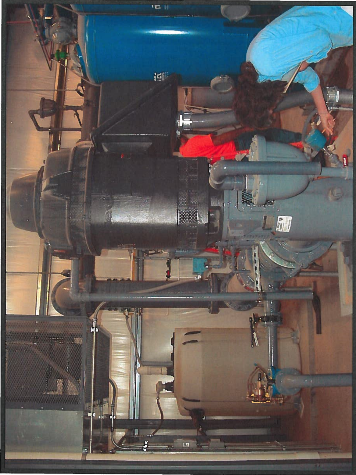
Well 16 Vertical Turbine Pump
