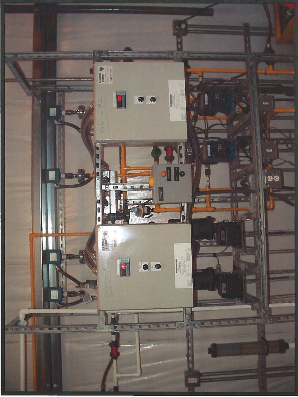
Chlorine Feed Pumps
