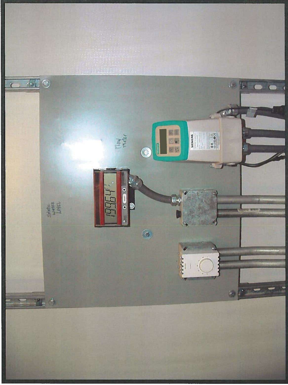
Static Water Level and Flowmeter Monitoring Systems
