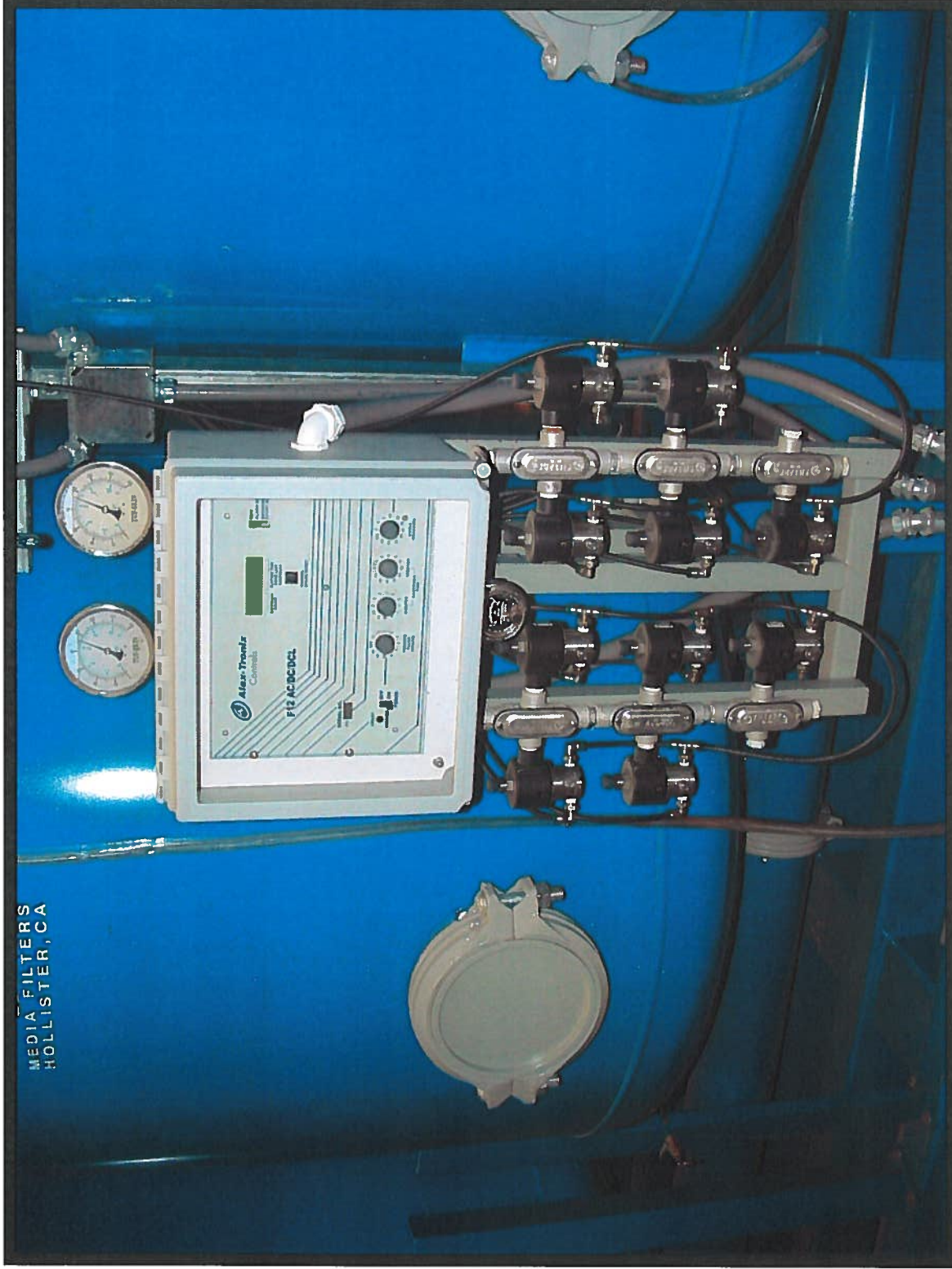
Filter Backwash Control
