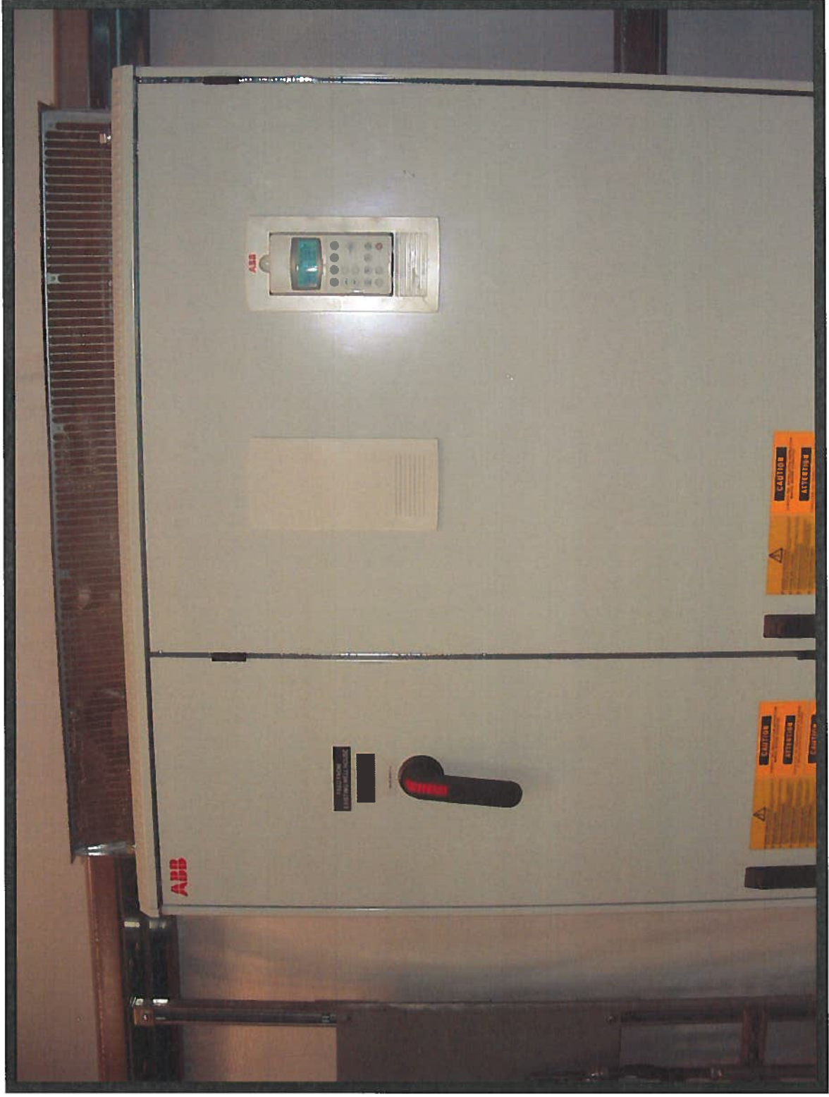
Well Pump VFD
