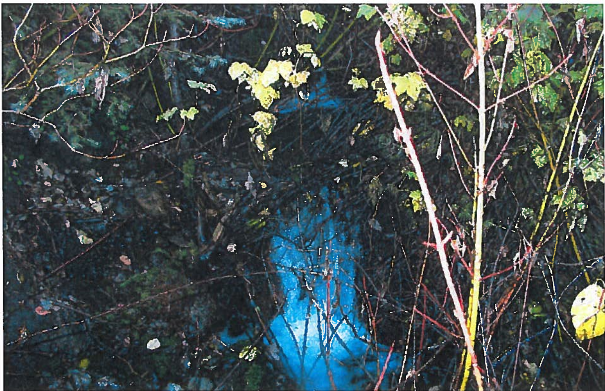
4. Allen ditch culvert outlet at West Mountain Rd. Very overgrown with vegetation.
