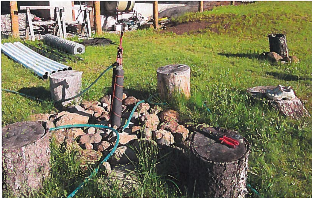
Irrigation System - standard garden hose and standpipe
