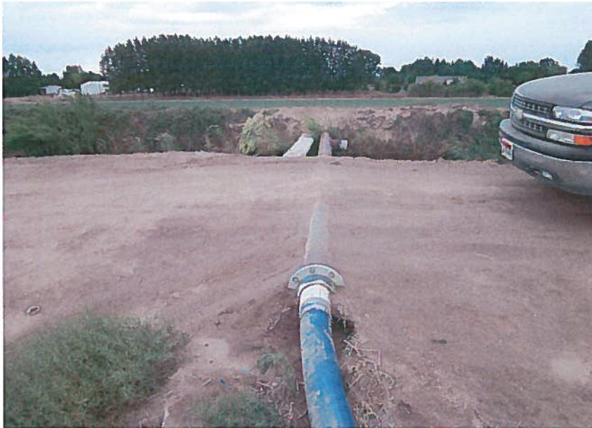
Pipe from well to west field for drip irrigation system.
