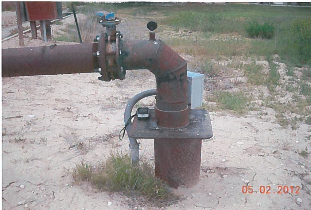
Well to 8" steel pipe. Pressure gauge seen. Well not operating day of exam.
