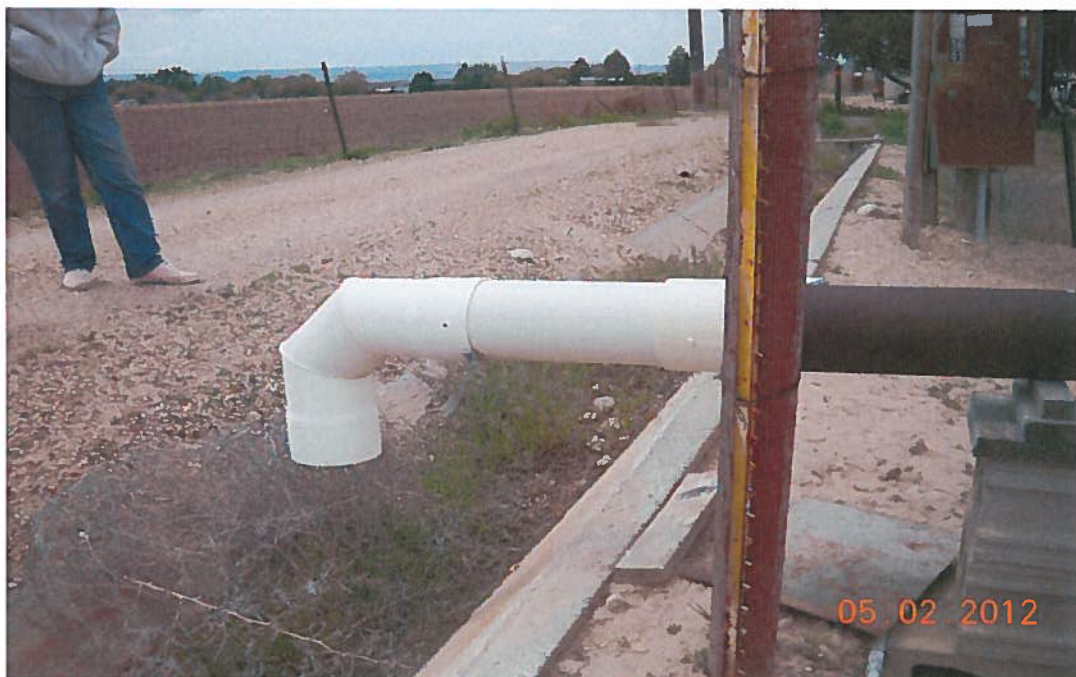
Steel pipe to PVC pipe to ditch which also delivers the Wilder Irrigation District water.
