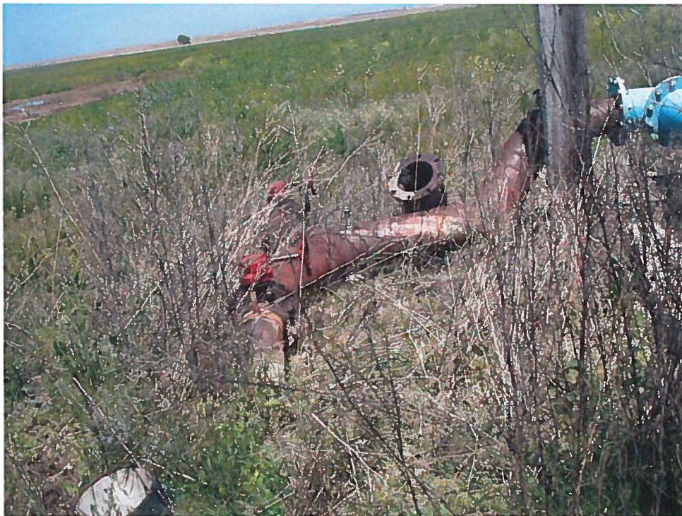
63-12421 Exam 5/14/2012: 6" mainline with shut off valves facing north. Blue 10" line from well to first "T" visible in upper right corner of photo. Well just outside right edge of photo.
