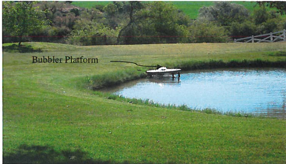
View southeasterly of river sewage pump discharging through a bubbler platform in irrigation pond. River sewage pump and irrigation pond submersible pump run simultaneously to maintain an approximate water surface elevation for the irrigation pond.
