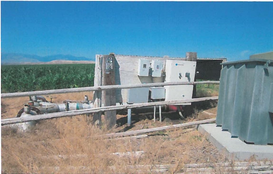
Well #2 is located at the center of the east pivot. The well ID was attached to the railroad tie just below the township/range sign.
