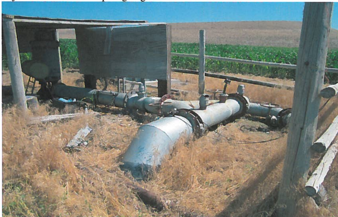
Well #2 was measured at the discharge pipe out of the well. The system T's with the right leg traveling east underground to Well #1. The left leg travels southwesterly underground to this pivot and on towards the western pivot.
