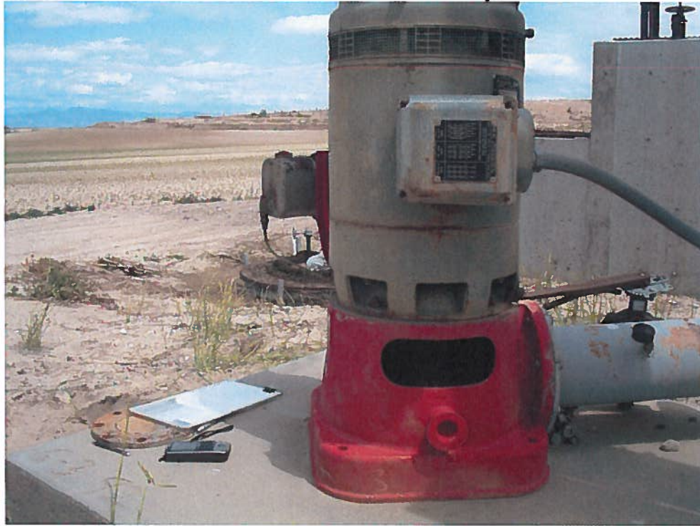
63-11722 Exam 5/22/2012: POD facing east/northeast. Surface water irrigation headgate box and "can" in background. 8" dia discharge line piped around backside of headgate box into "can" to 6" buried lines to pivots.
