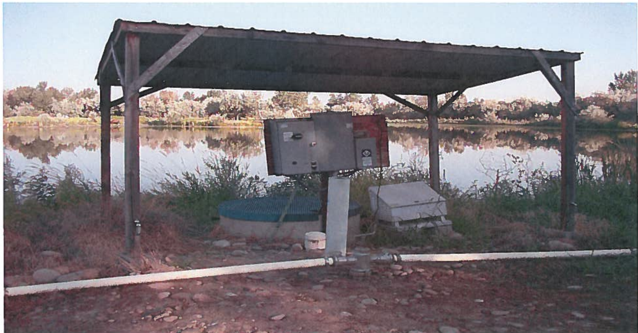
POD – Irrigation Pump , photo #1 on exam diagram map. Shallow ground water cistern, submersed pump. Control panel seen, flowmeter in upright light blue standpipe, 3" surface lines in foreground (4" main from pump is buried). Lockable blue grate covers top of cistern.
