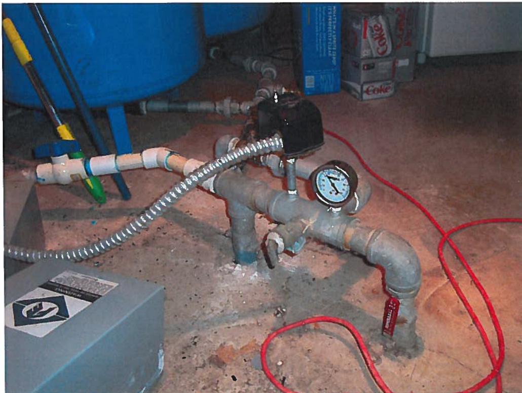
63-12001 Exam 5/17/2012: Pressure gage inside garage on line from well to home, gage before pressure tank. Likely same pressure from well into irrigation mainlines.
