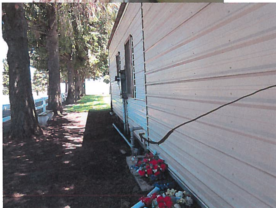
Pipe comes from well to pump house
