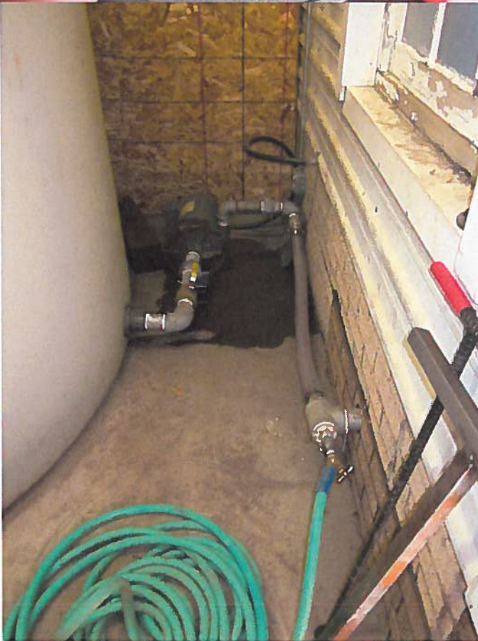
Pipe conveys water from storage tank to irrigation system
