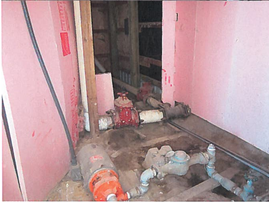
10,000 gallon Storage tank behind the wall
