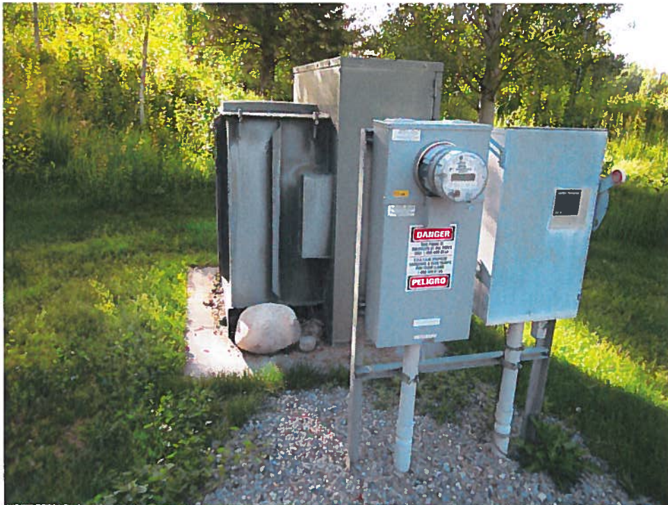
Electrical Box for pump house
