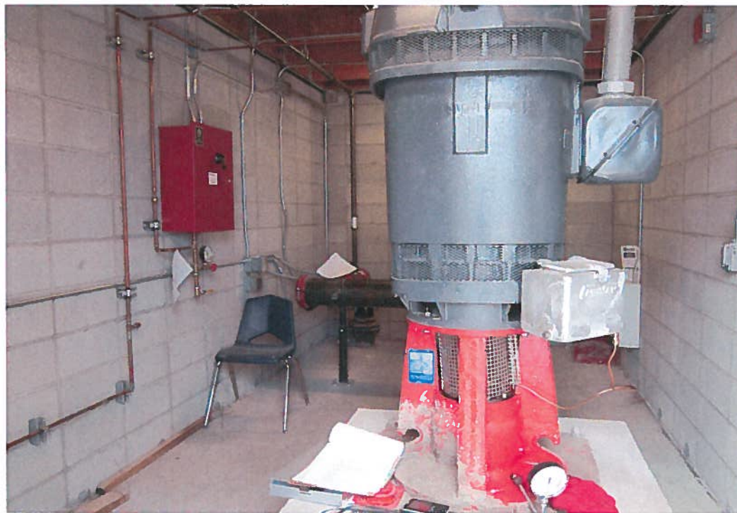
Both photos are of the fire protection well and motor in riser room on north side of 8 th grade building.
