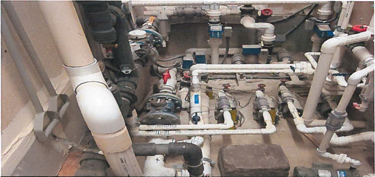
Place of Use: View inside of home of waste water mechanical room distribution piping and pressure and flow controls.
