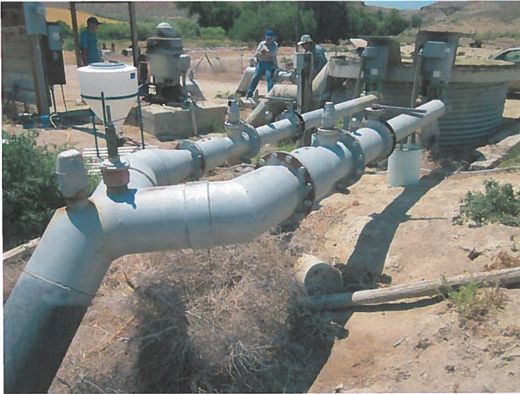
This photo shows the two booster pumps supplying water to the north fields.
