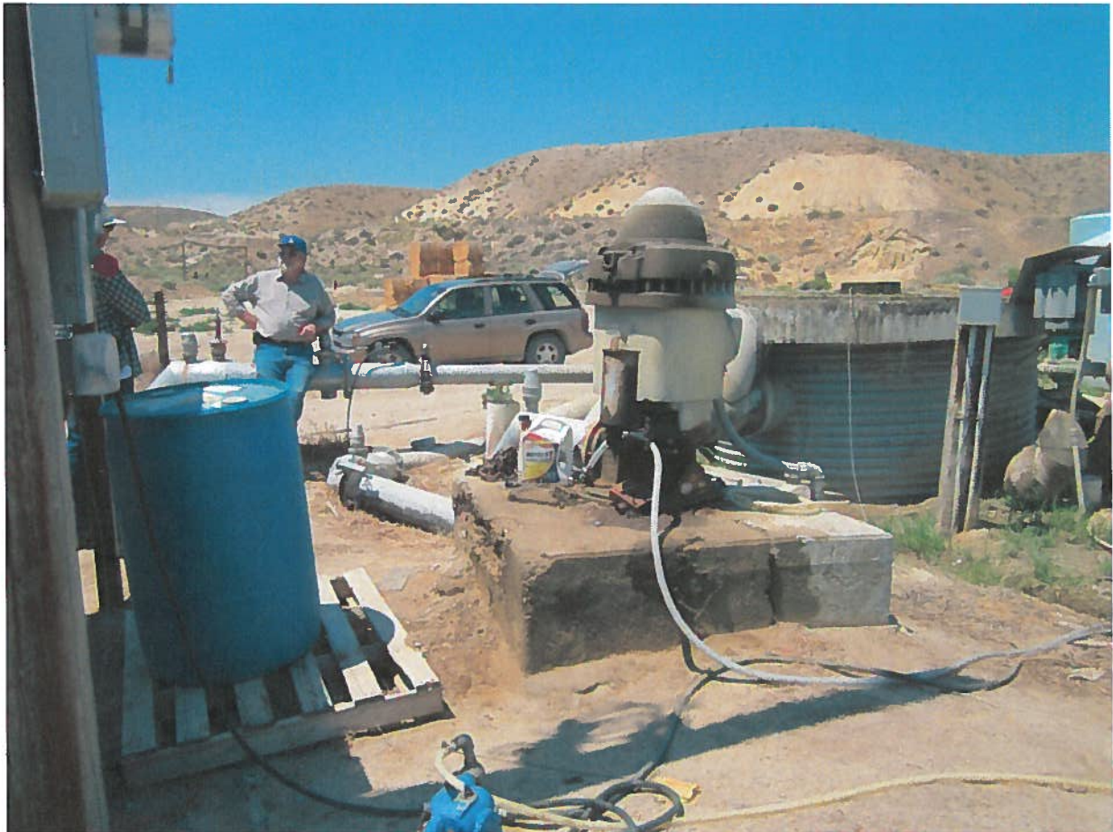
This photo shows Well #1 (A0016967) next to the holding tank. The pipe at waist height with the vehicle behind it has a 50 hp booster pump attached and supplies water to the field south of Sinker creek.
