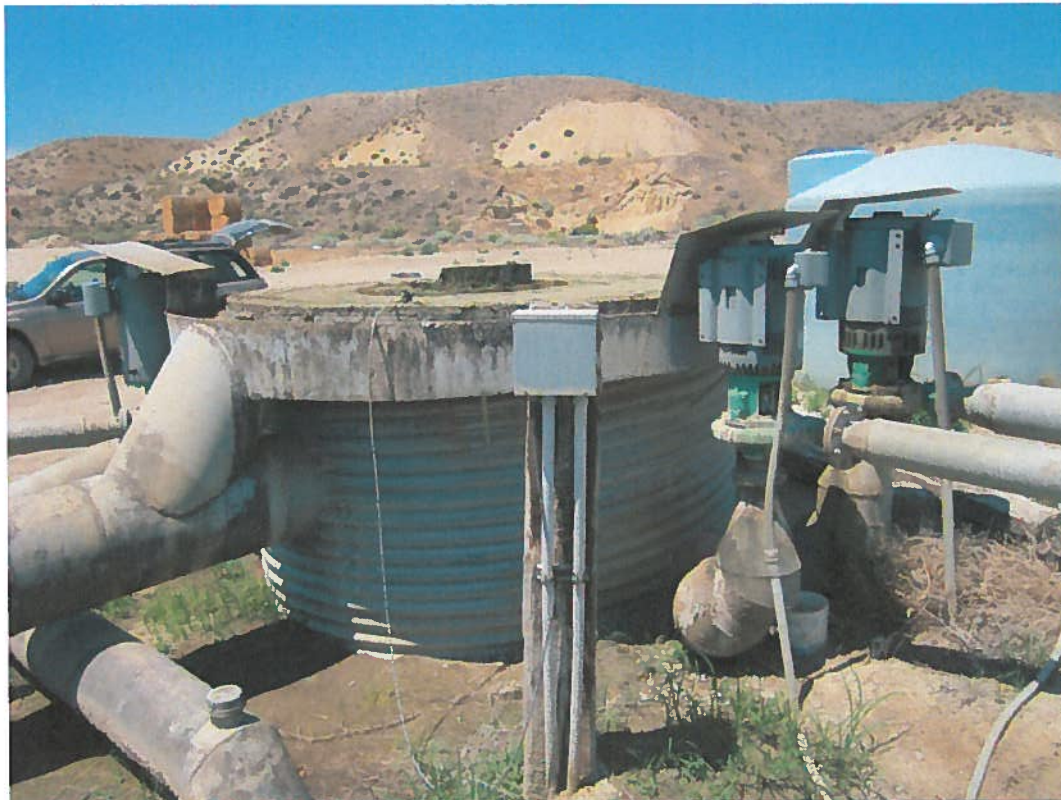
This photo shows the overflow pipes on the left. The two booster pumps on the right supply water to the pivot and fields north of Sinker Creek. The pump closest is a 25hp, the pump with the blue fertilizer tank behind it is a 50 hp.
