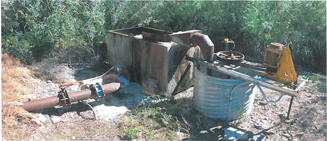
Irrigation pump which pulls water from Snake River and supplies fields south of pond.
