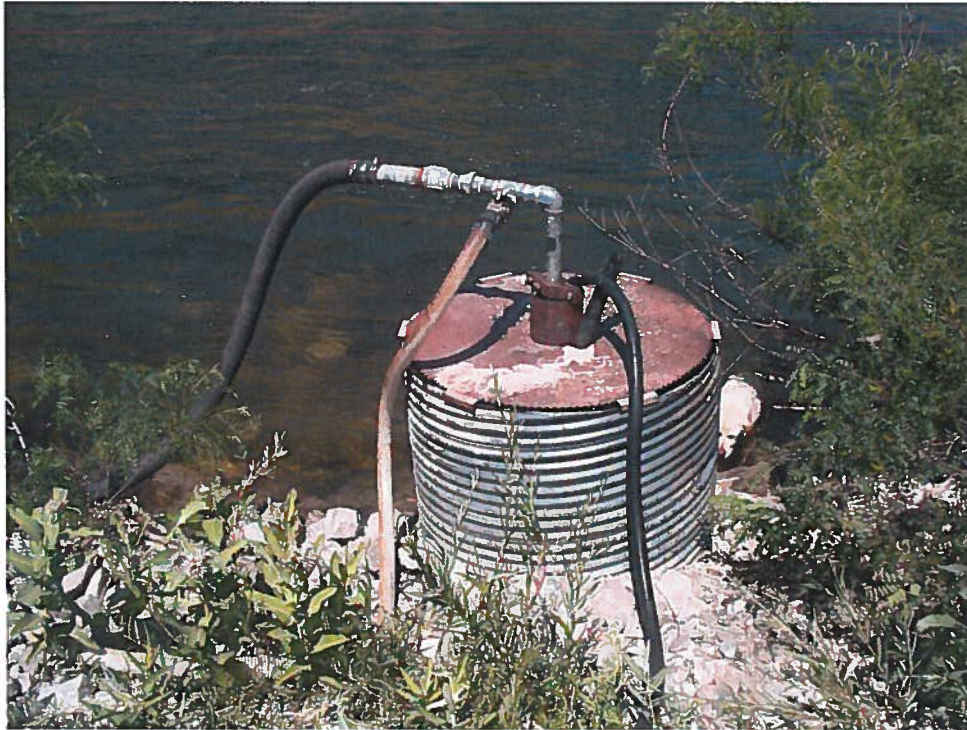
65-22659 Exam 7/30/2012: P/D facing north. Pump inside corrugated pipe in river. 2 in diameter black hose/line leads to buried 4" PVC line to pump house and property to the south.
