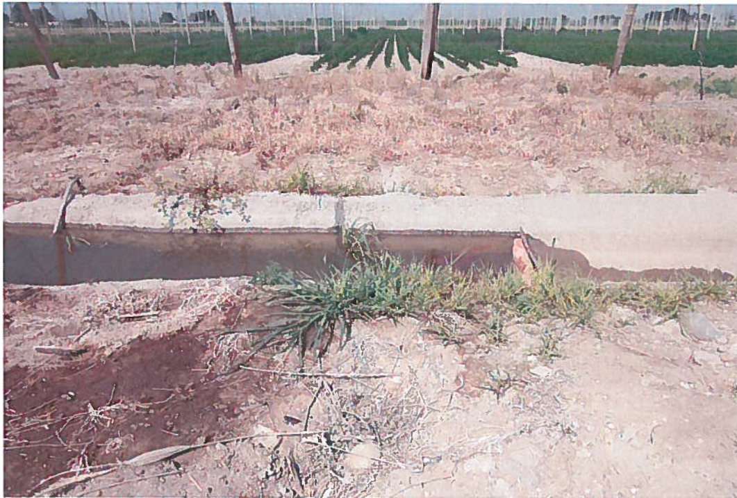
Place of use and portion of concrete ditch delivery system.
