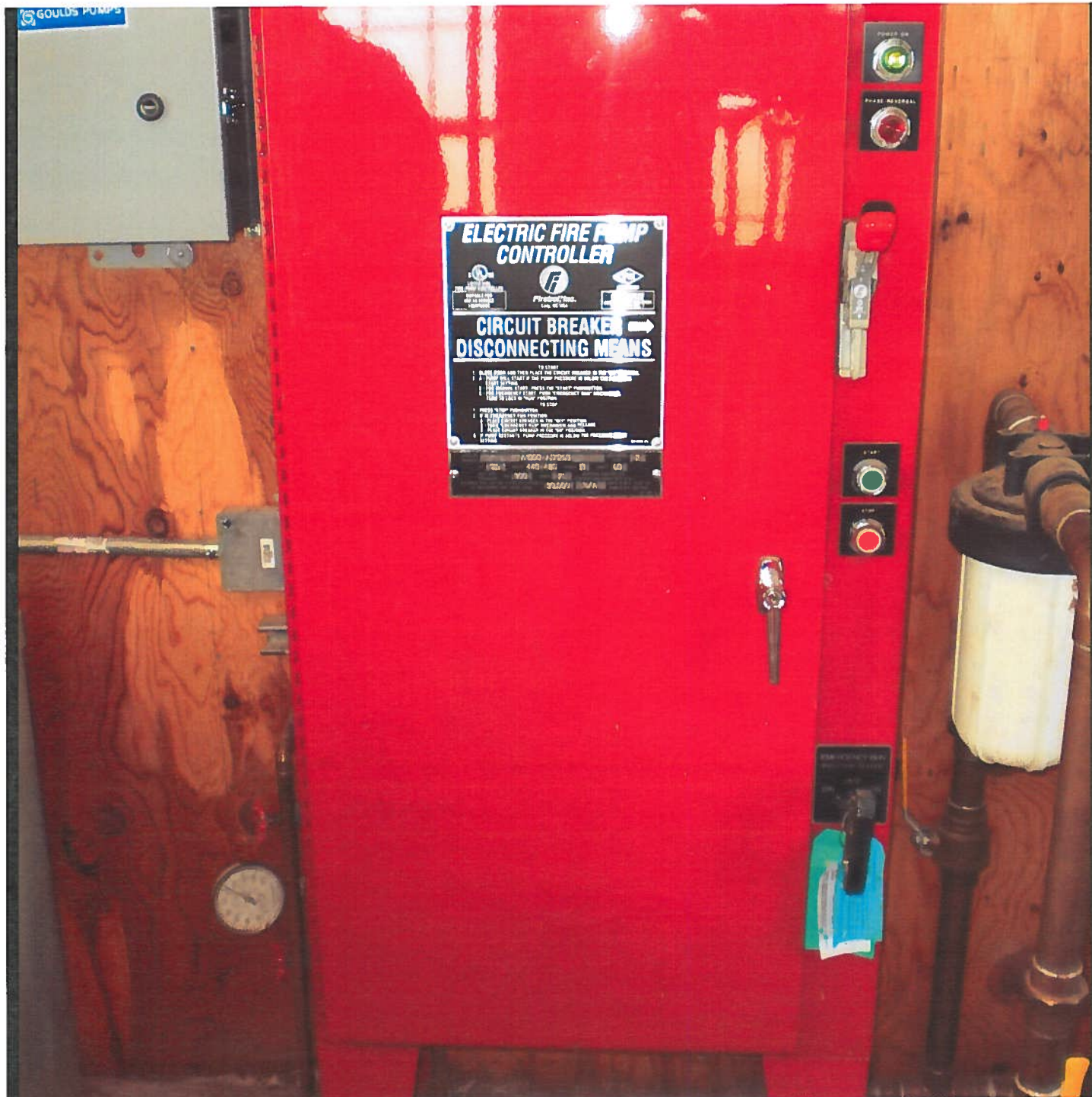
Fire system controls
