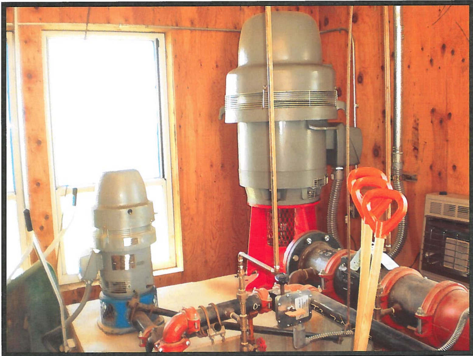
Fire system booster pumps
