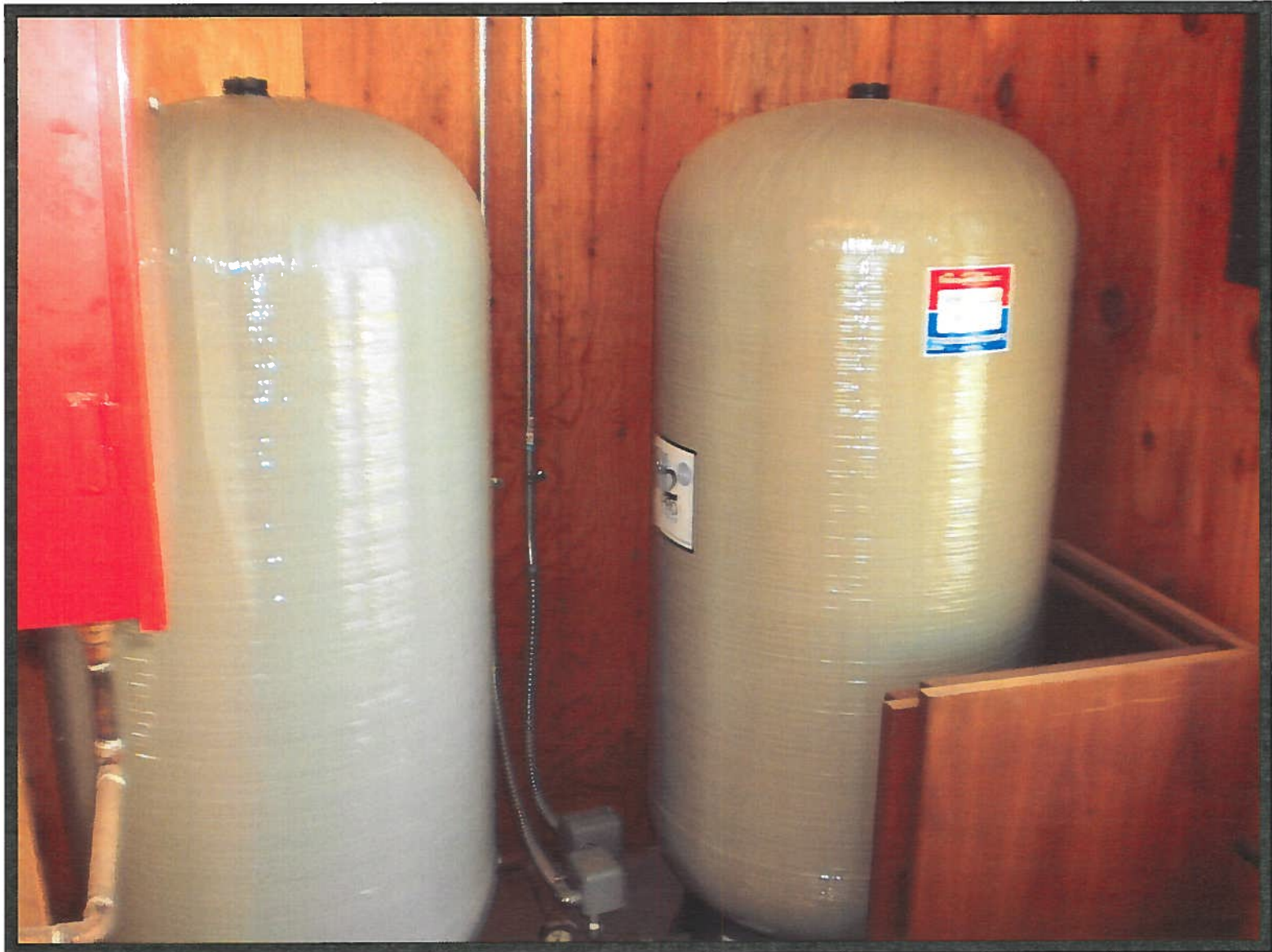
Domestic system pressure tanks
