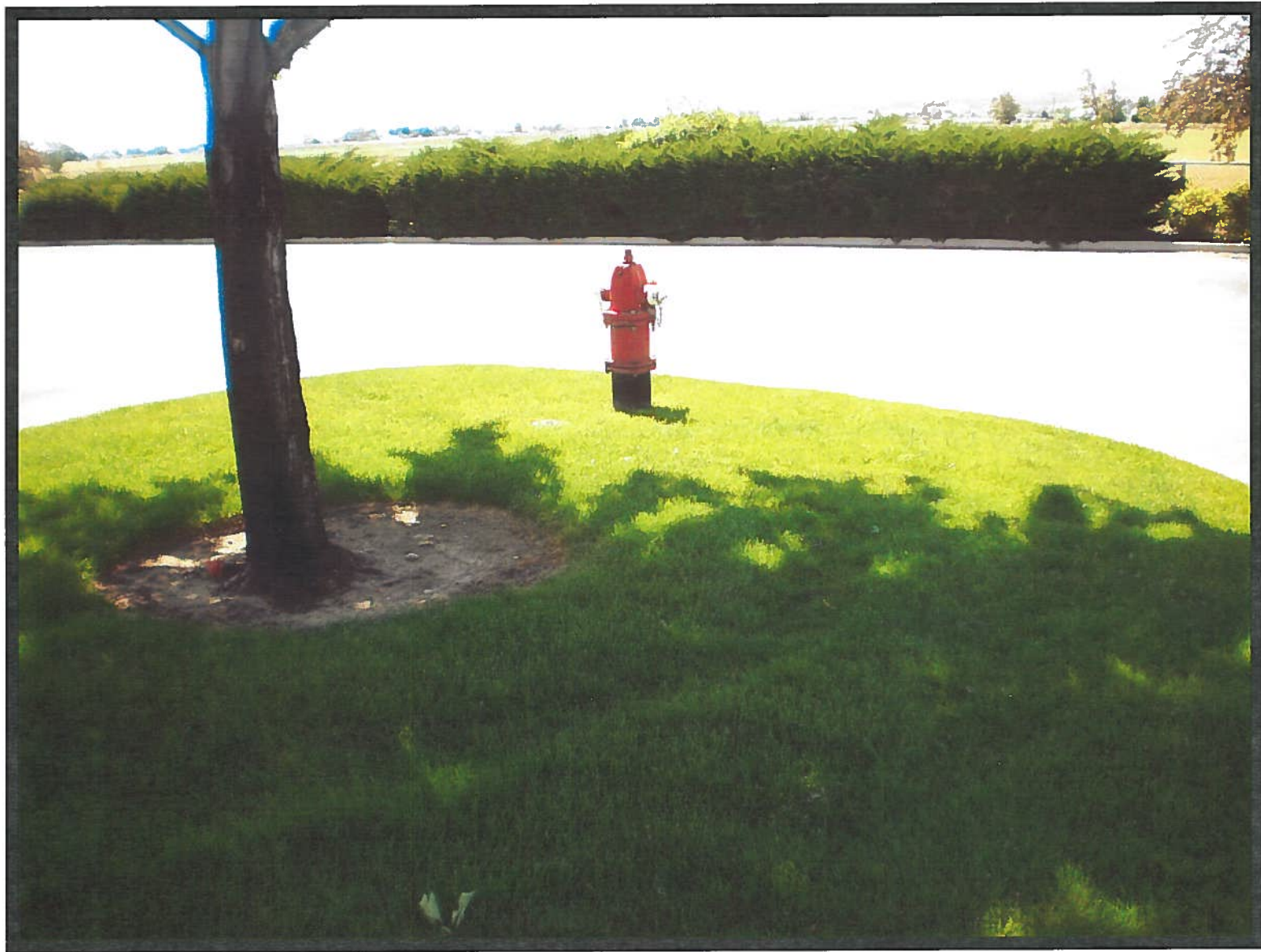
One of three fire hydrants
