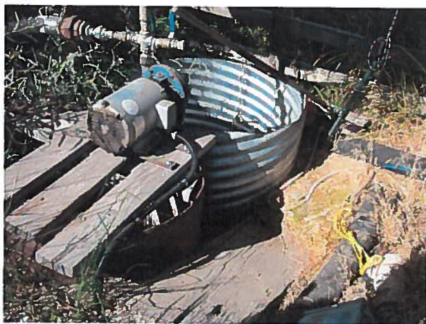
Pump and motor, 1 inch discharge on top of pump
