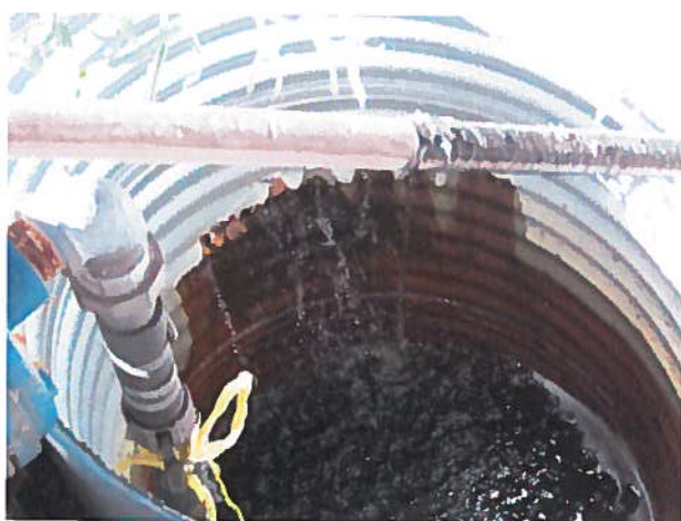
Sump (culvert) collecting waste water from irrigation
