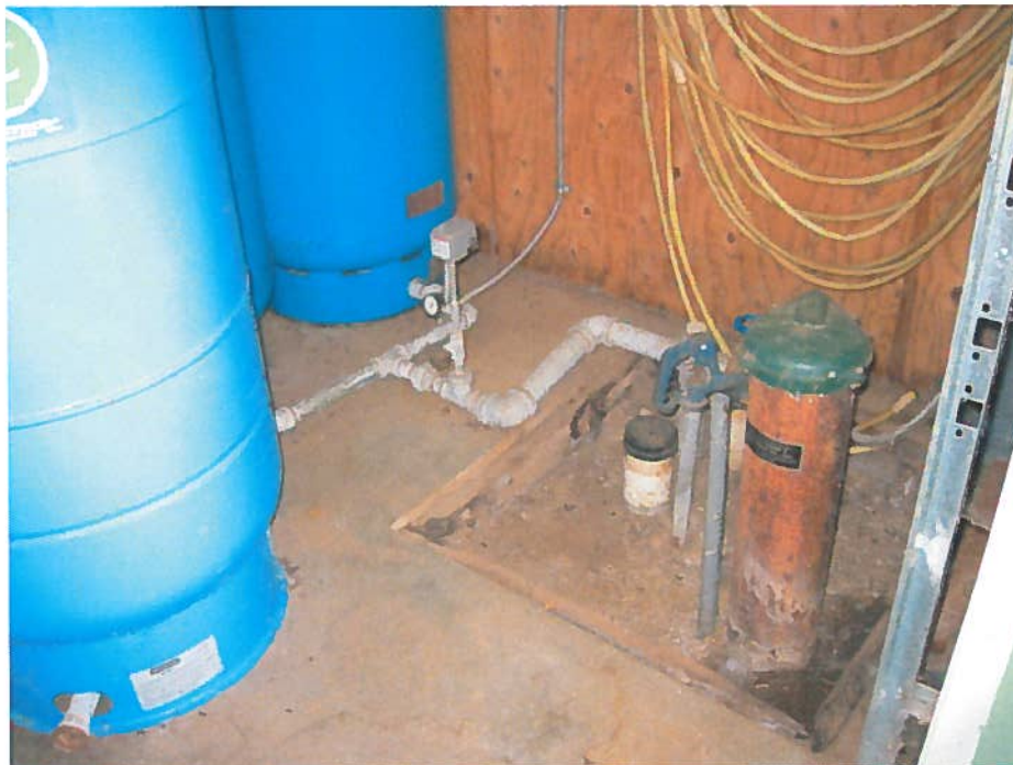
North well feeds 2 tanks. Tank on left forward, not connected. This is a 3 HP pump as indicated by the tag on the power distribution panel.
