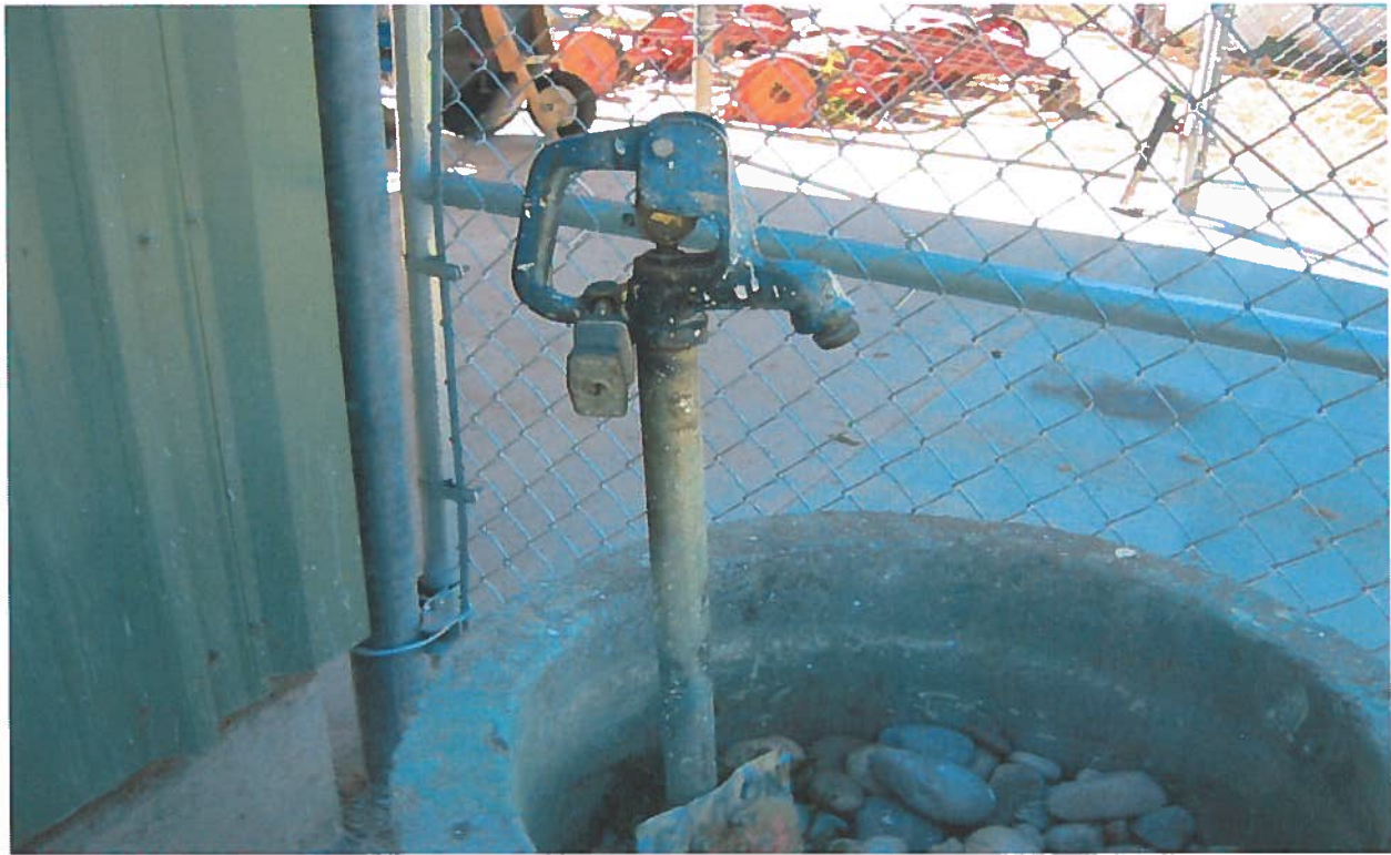
"Bury" hydrant located next to maintenance shack with a standard \frac{3}{4} inch hose nozzle.
