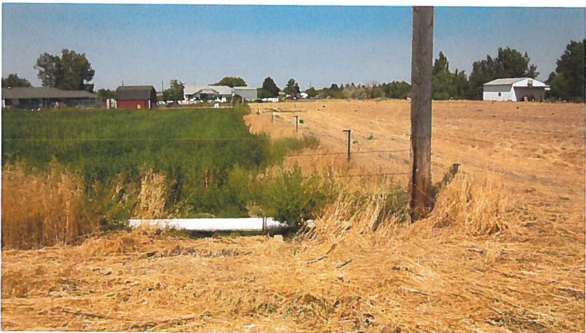
Second riser pipe – Continuing west on Grandview Road from the above picture, looking north at the second riser pipe for the irrigation system approximately 110 feet west of the diverter.
