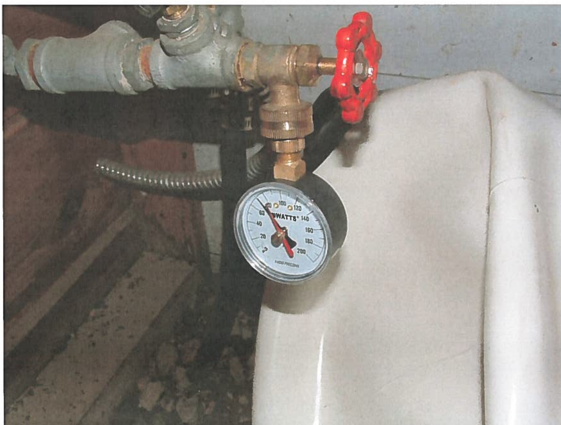
80 psi discharge pressure measured at cottage while sprinklers were operating.
