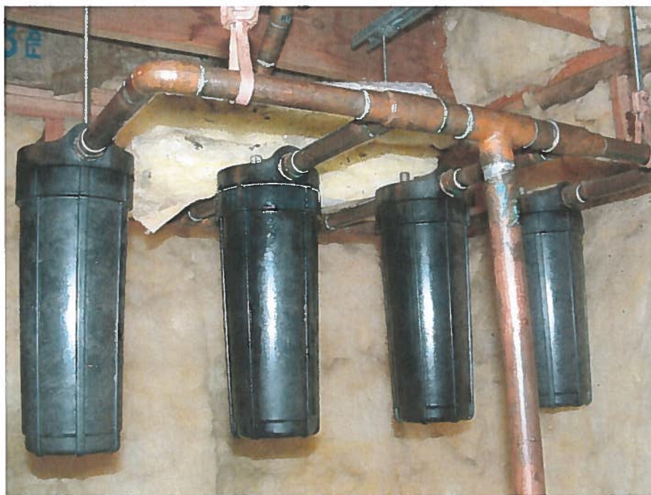
Filters on discharge from pump.
