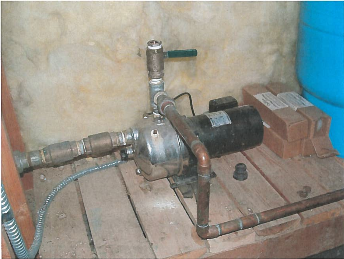
Grundfos jet pump and motor located in basement of house.
