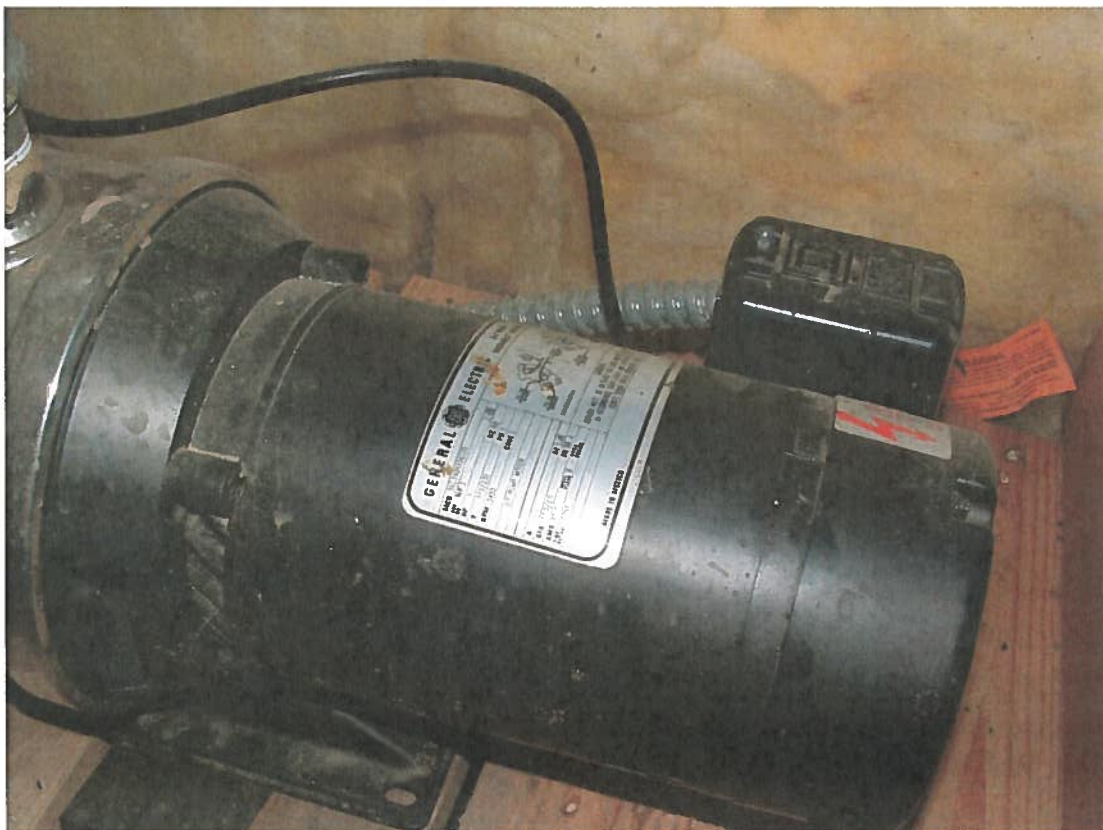
1 hp jet pump motor.
