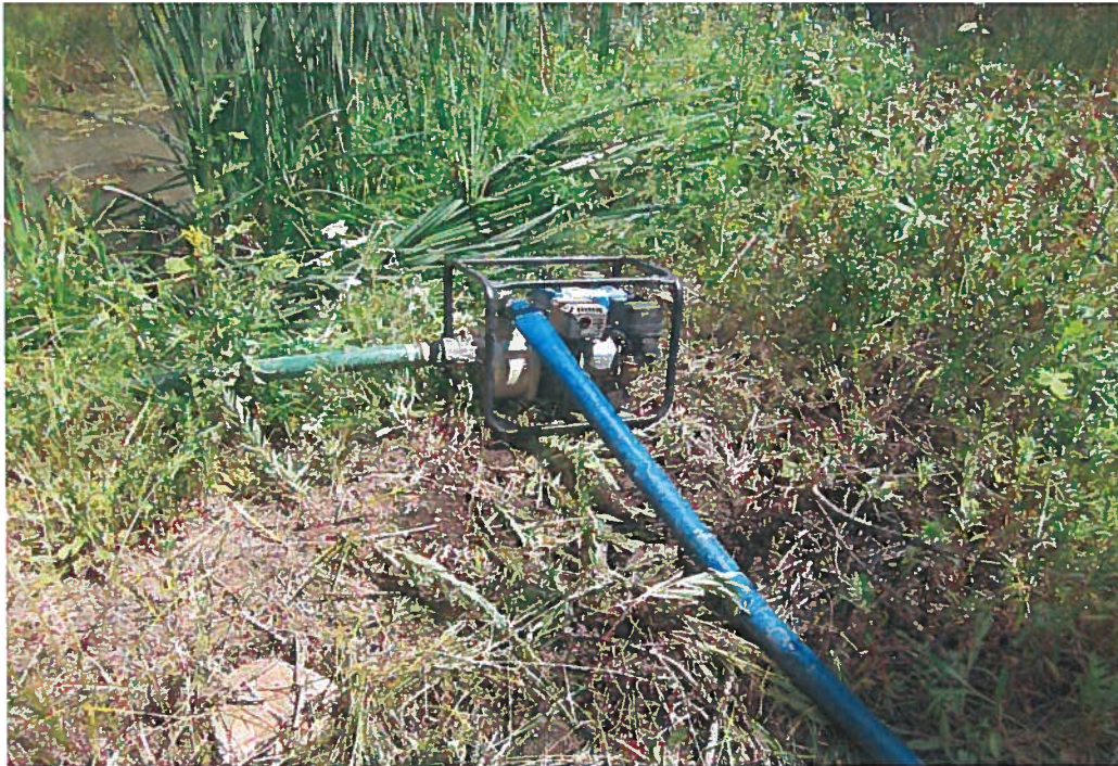
POD – pond seen left back. 6.5 hp motor and pump diverting through 2" hose from creek.
