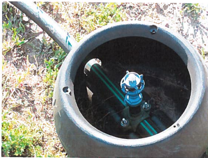
Nelson Rotor sprinkler pod. All sprinklers used in the distribution system are of this type.
