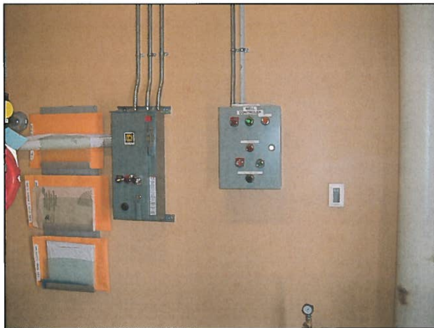
Figure 8: Well pump controller and switch gear.
