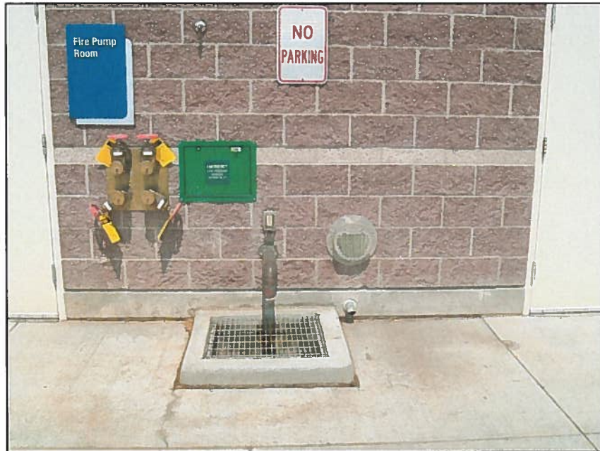
Figure 7: Flush flows are discharged outside of operations building into a collection box, and then to a stormwater basin.
