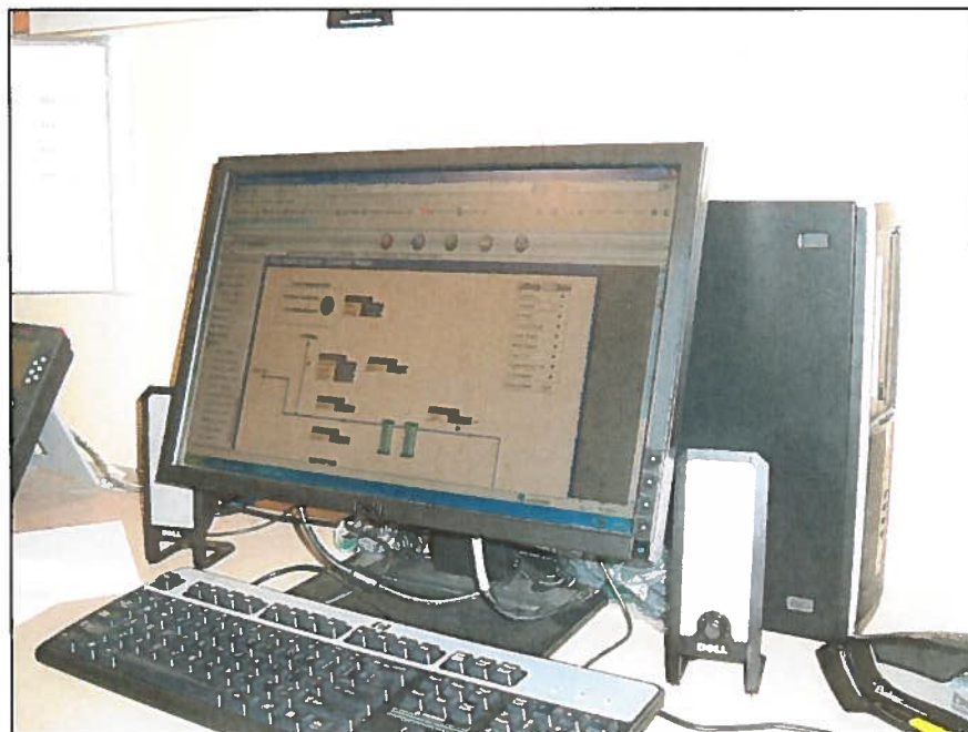
Figure 10: Emergency water supply operating system interface.
