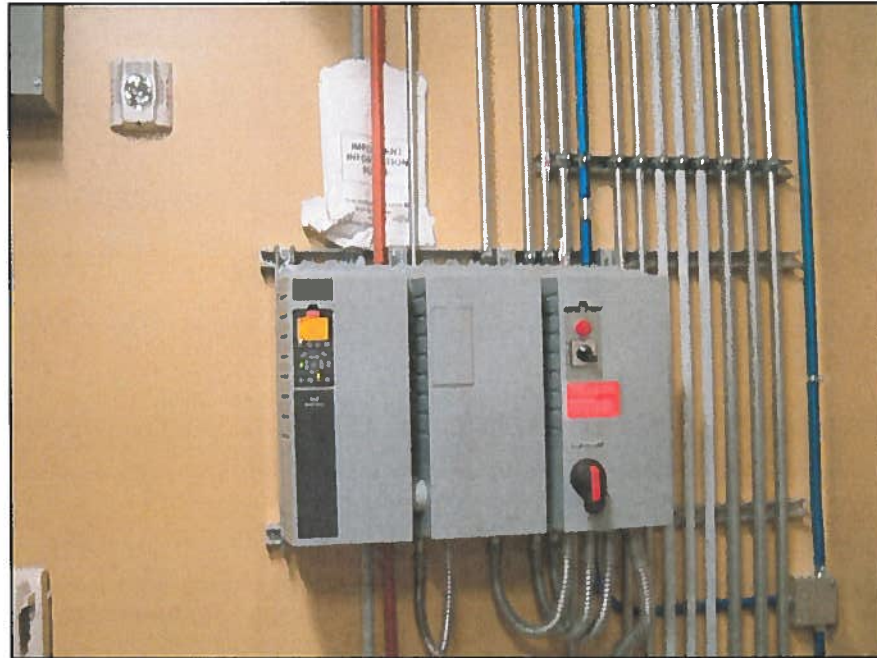
Figure 9: Well pump variable frequency drive.
