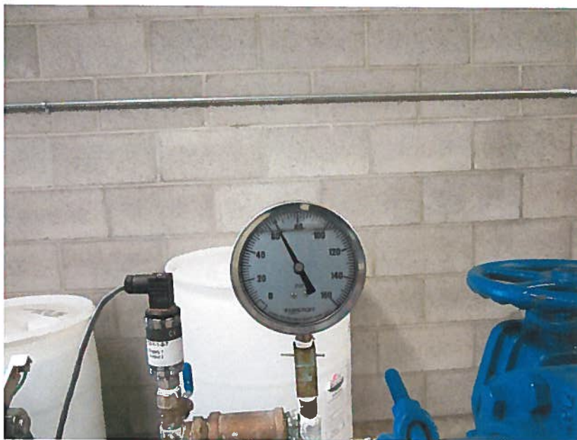
Photo 1. View of the pressure gauge on Well #6. Photo taken by D. Owsley on 8/9/2012.
