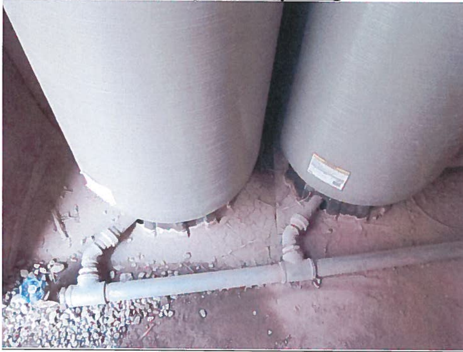
Picture of pressure tank plumbing
