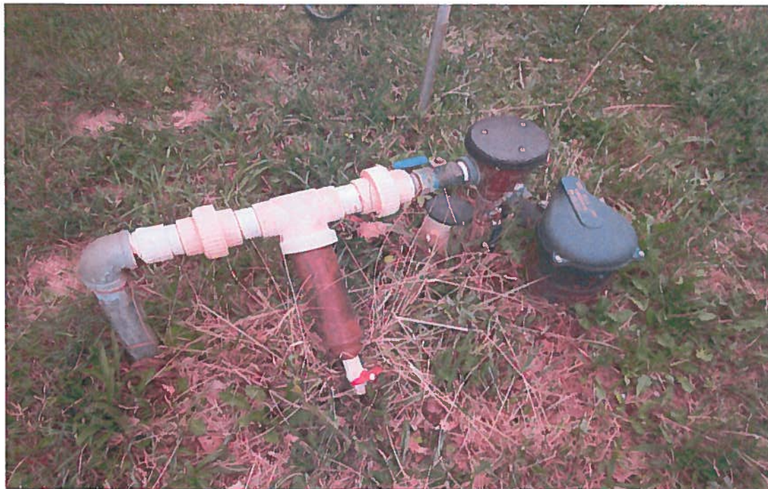
Point of diversion = well, which is fitted with a 3 hp submersible Gould pump and motor.
