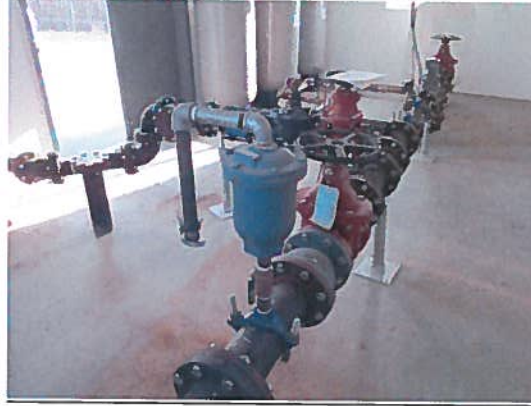
Picture inside Well House
