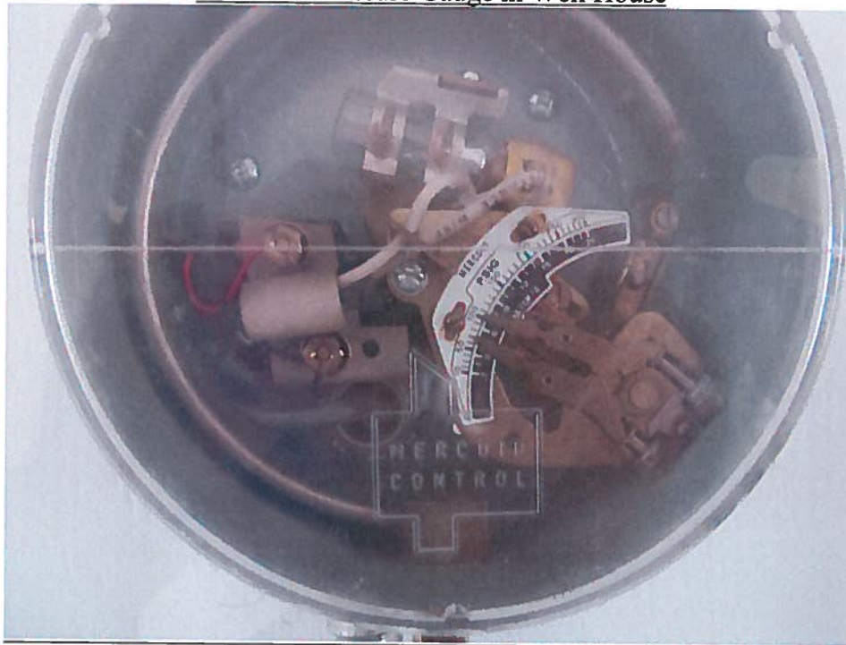
Picture of Pressure Gauge in Well House
