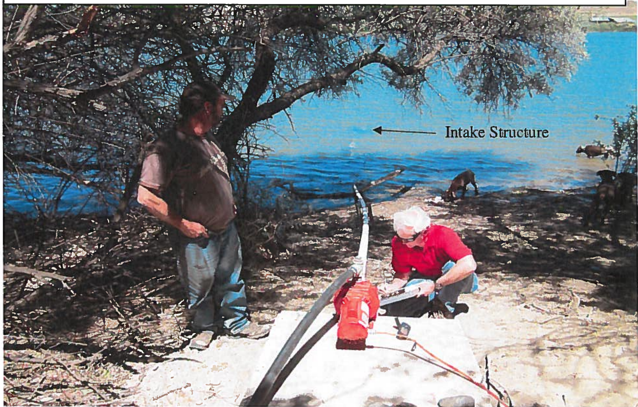
Point of Diversion: View northerly of 2" PVC suction line to submerged intake structure (barrel), 2 hp pump, and 1 1/2" PVC discharge line.
