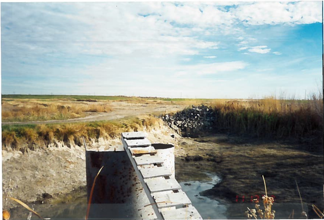
Pond For Canal Water, Pump Inlet
