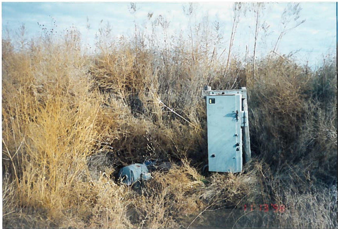
Pump For Canal Shares
