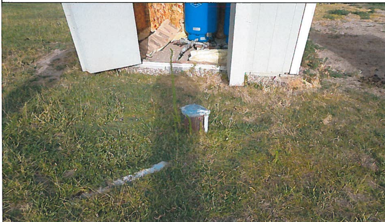
Point of Diversion: View westerly of well and pump/control house. The two pressure tanks in the pump/control house are for domestic use in home.
