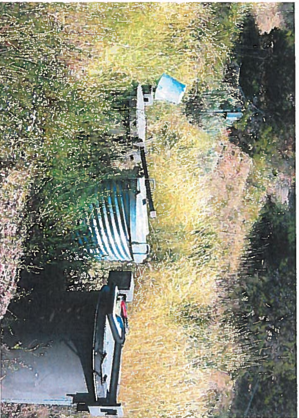
Water Facilities at Mink Cr. Campground
