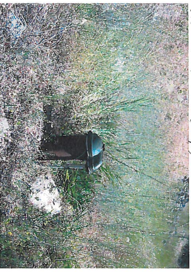
Wellhead - Mink Cr. Campground
