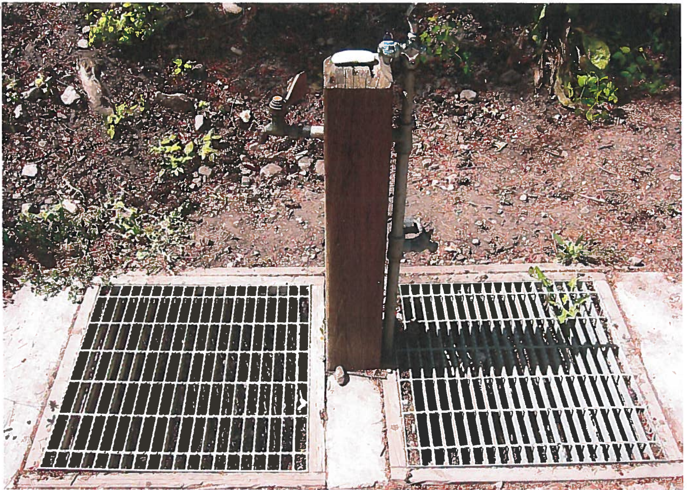
Hydrant/ Faucet/ Drinking Fountain system
