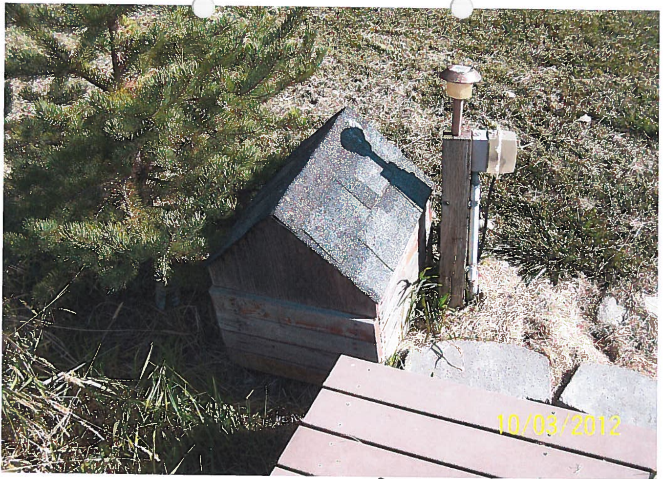
Electric Pump, in the event of Fire Protection.
