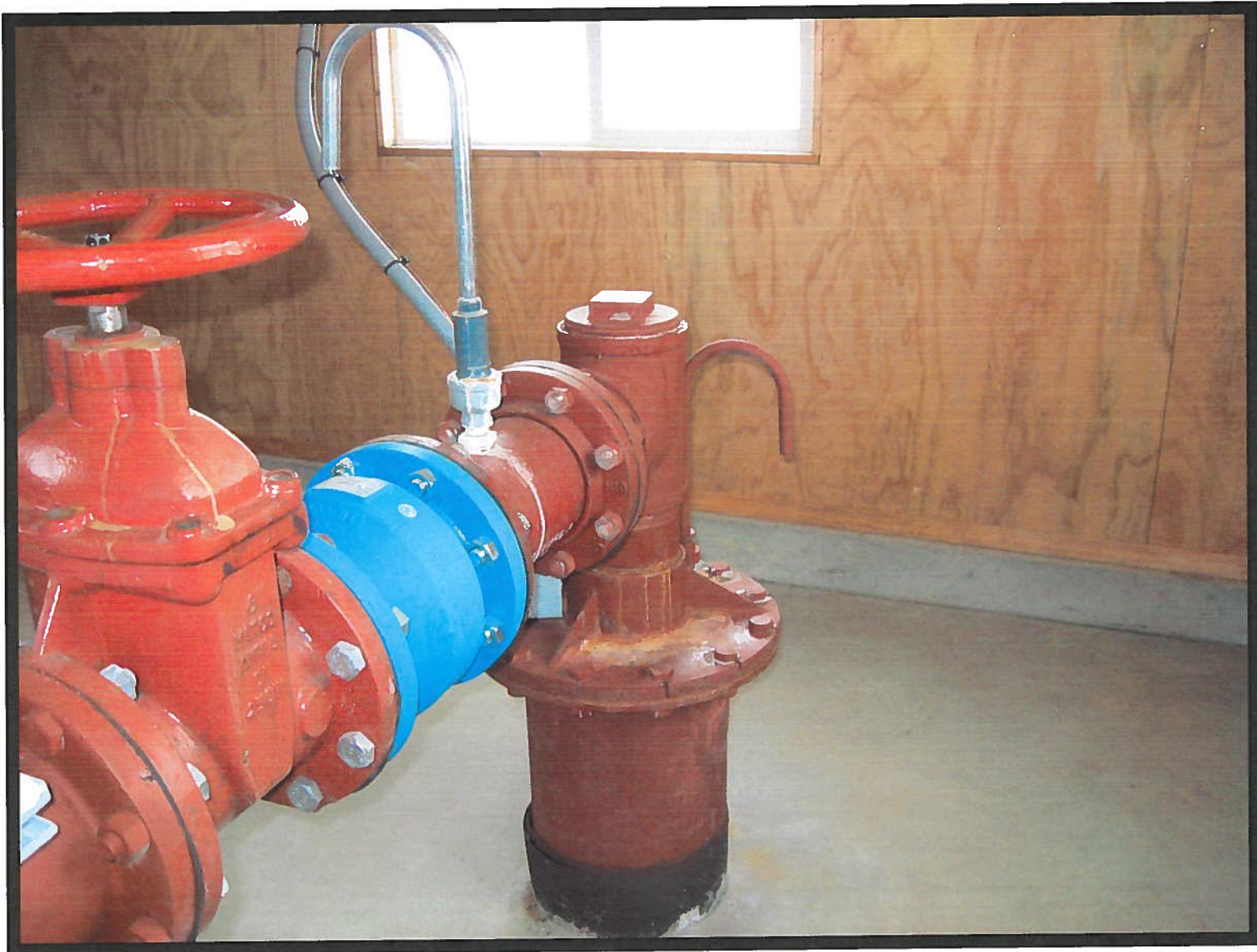
Back-up Well No. 1 Located Inside the Well House
