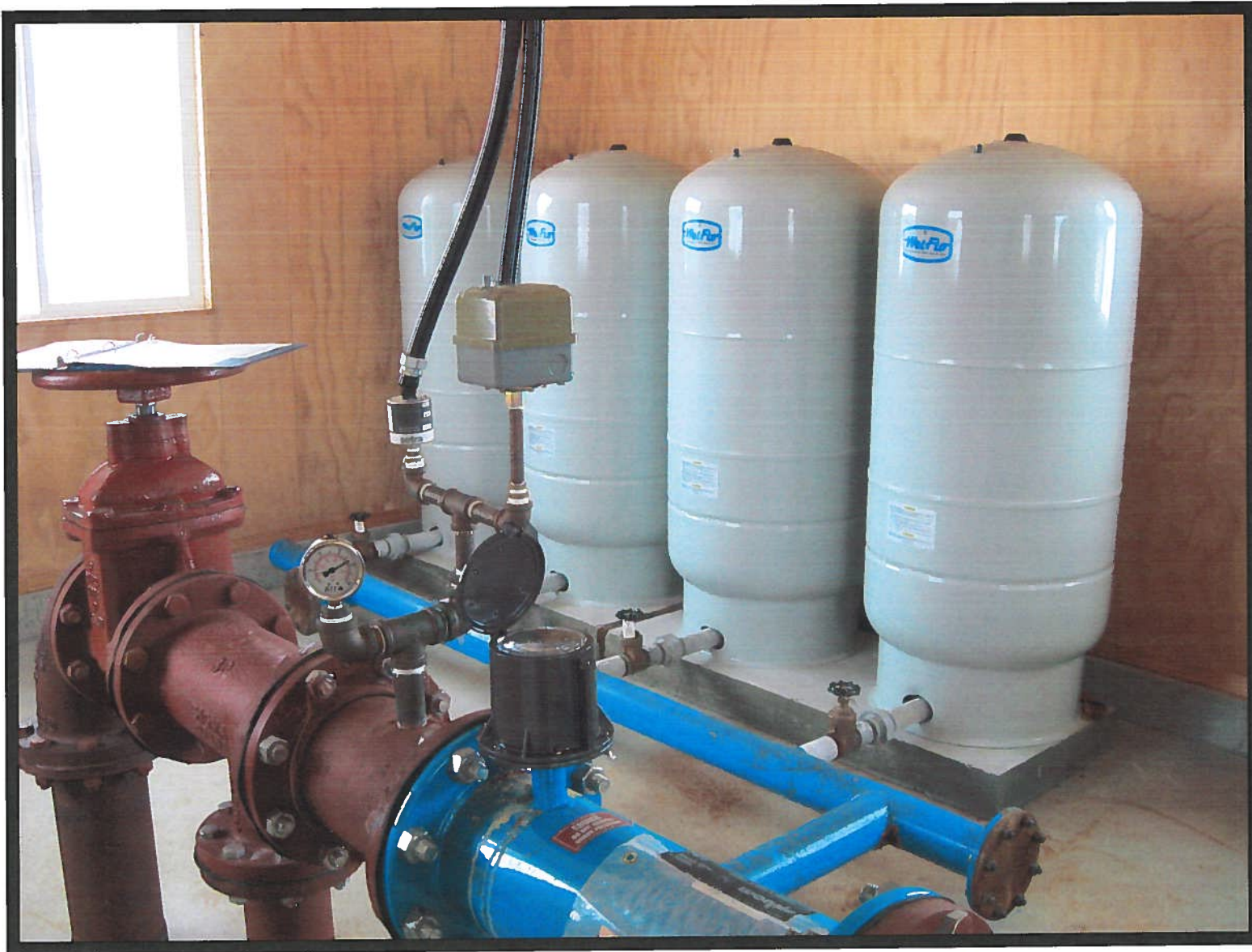
McCrometer Flowmeter, Pressure Gage, 135 Gallon Storage Tanks
