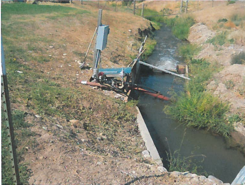
Photo of the POD. Pump was not running at the time of the field exam.
