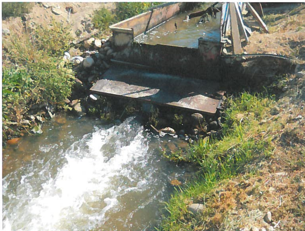
Downstream looking up at the pump.
