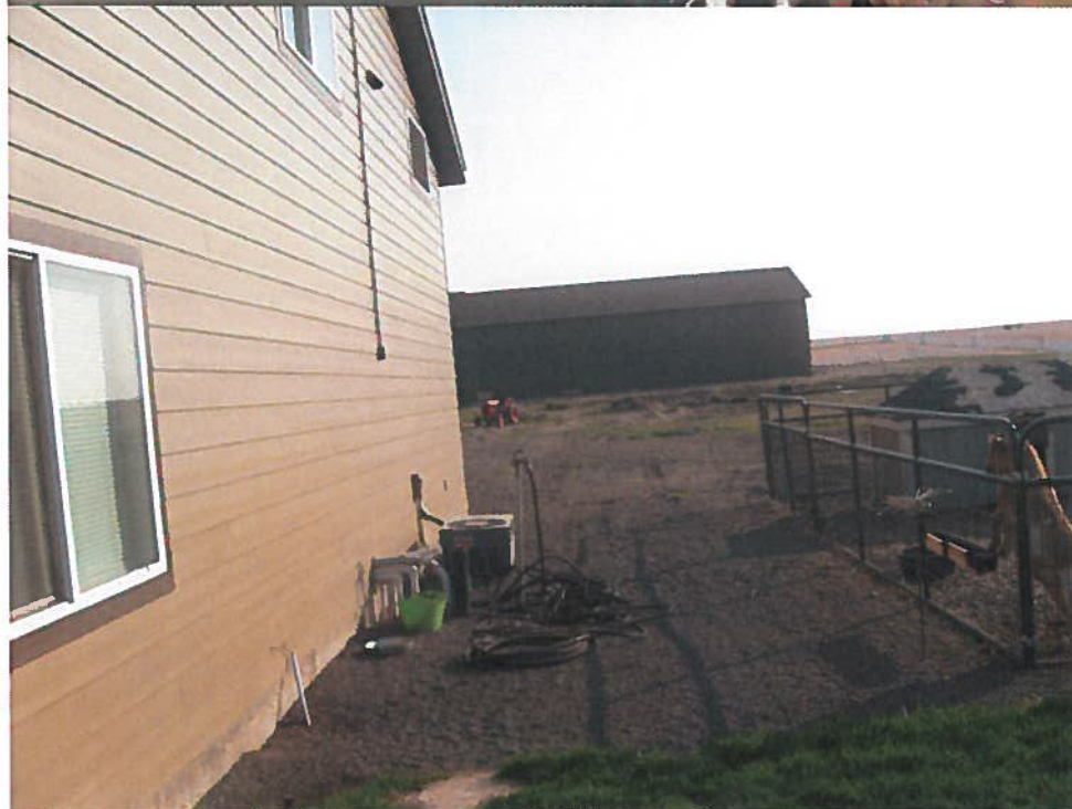
Hose and hydrant on the west side of the shop.
