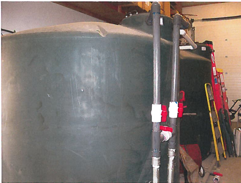
2 - 2500 gallon storage tanks
