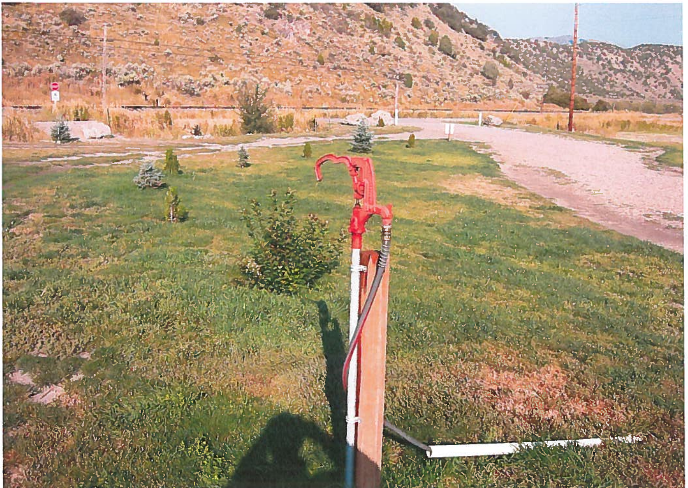
Nydrant at RV Park
